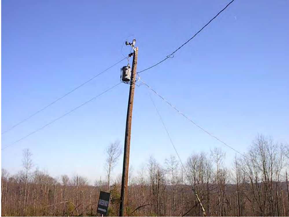
Fig. 5.6. Pole-mounted transformer at a city of Oak Ridge water tank at Parcel ED-6.
