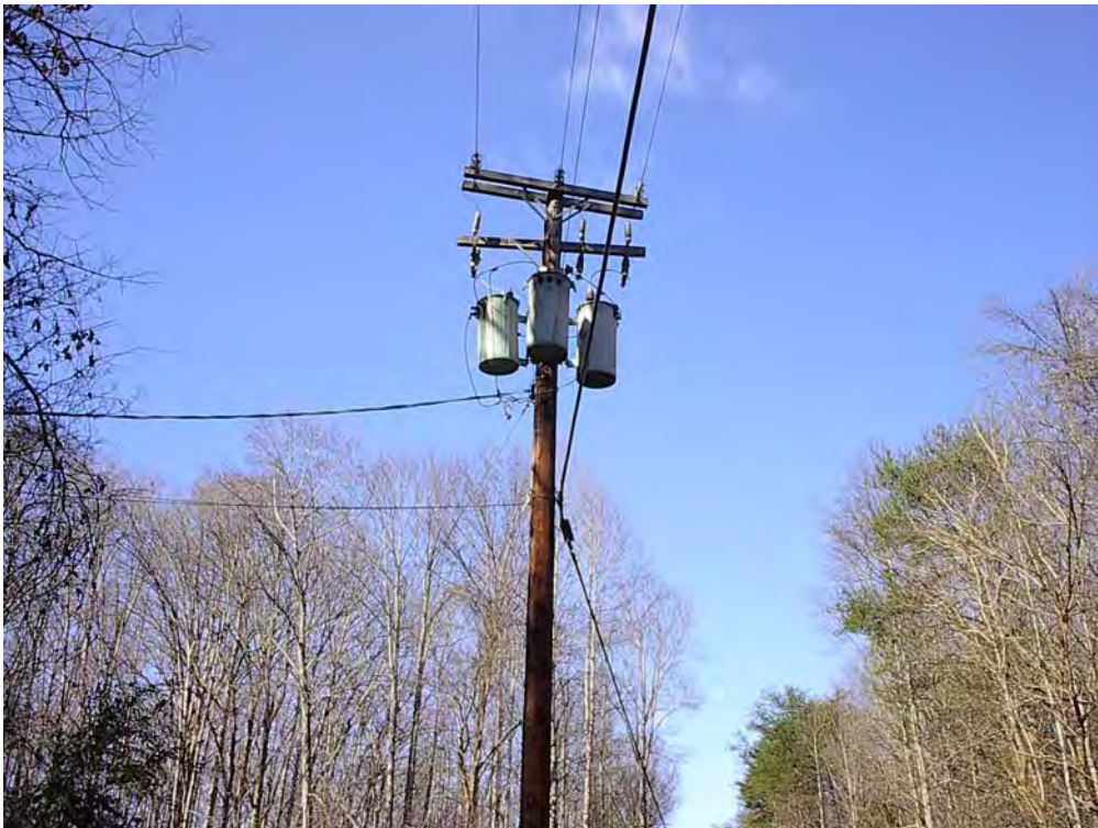
Fig. 5.7. Pole-mounted transformers at the city of Oak Ridge pumphouse at Parcel ED-6.
