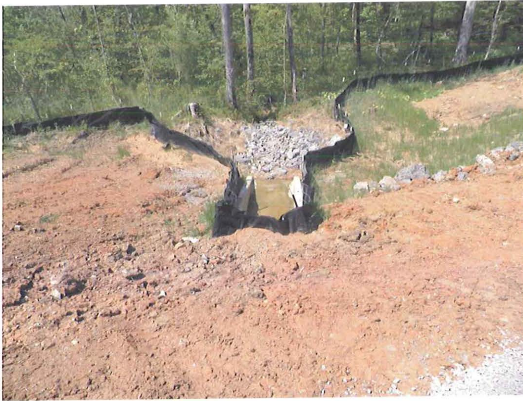
Photograph 5. View of drainage outfall in SR 95 ROW adjacent to Parcel ED-1 NA boundary.
